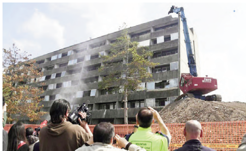
Fig. 12, 13 | Residence Garibaldi 2: the renovated block 3; the demolition of blocks 4, 5 and 6 to be replaced with trees, a basketball court and a children's play area (credits: Comune di Calderara di Reno, courtesy of P. Zullo, 2019; Photo Schicchi, 2019).
