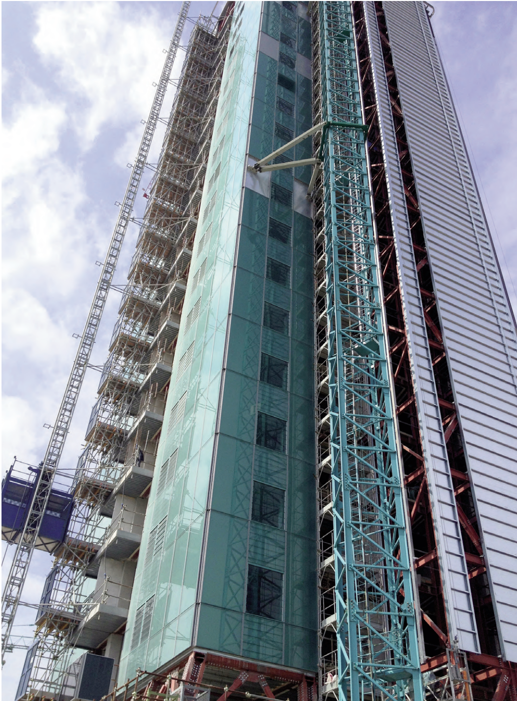
Fig. 5 | Residential Tower in Castelmaggiore (Bologna), during the construction phase of the double-skin glass facades. Building's general features: 7,000 sqm of built surface, n. 90 apartments, n. 1 commercial structure, n. 1 restaurant, n. 1 Spa, offices (credit: F. Conato and V. Frighi).
