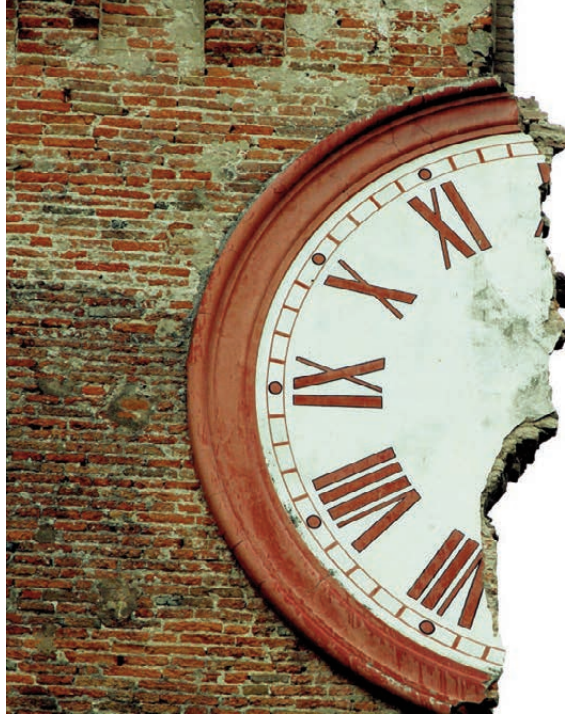
Fig. 6 - The Clock Tower in Finale Emilia (northern Italy), after the earthquake in May 2012 and subsequently entirely collapsed (credit: http://i.imgur.com/TqSgJ.jpg ).
