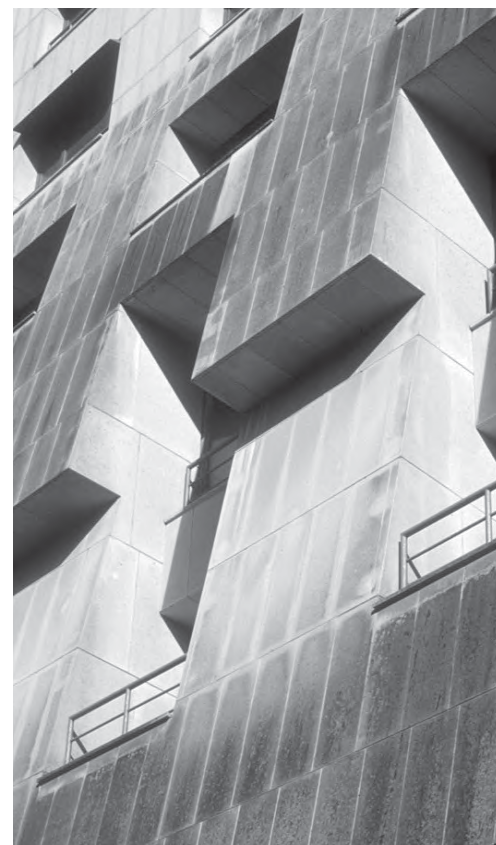
Figg. 5, 6 - From the top: L'Arche de la Defense (Von Spreckelsen, 1989) in Paris, separation of coating parts (by the Author); American Center (Gehry, 1994) in Paris, detail (by the Author).
